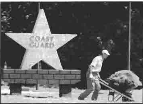
GETTING PREPARED — A worker places sod in the Veterans Memorial Park in preparation of its dedication October 14.
